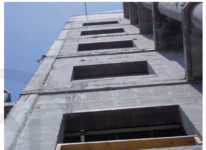
Fig. 4.4.3—Variations of concrete frame and masonry infill surface that is to receive plaster.
