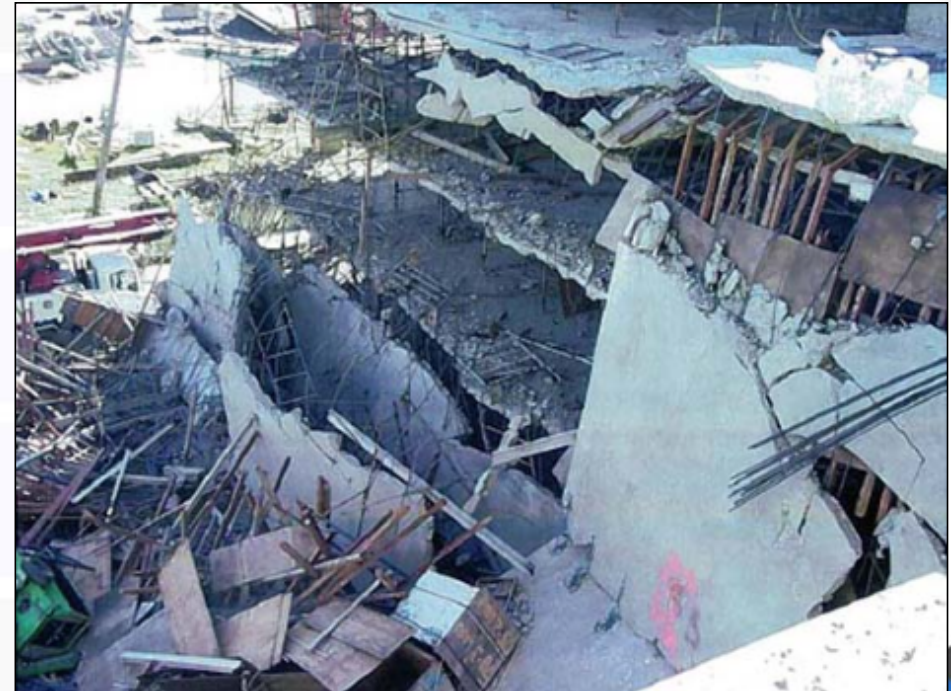
Berkman Plaza 2: Jacksonville, FL December 2007 1 Dead, 21 Injured
